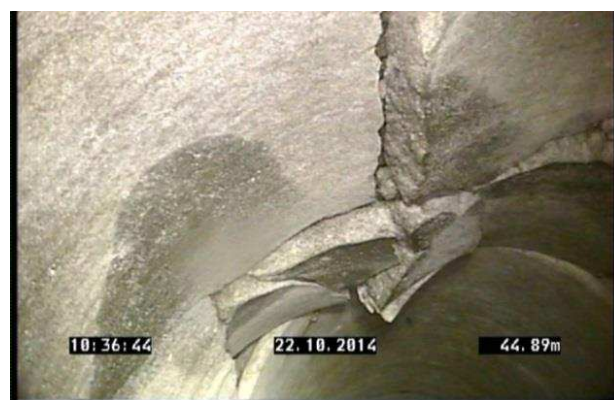
Image taken from a CCTV survey of a cracked and failing asset
